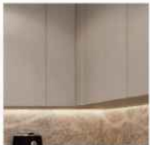
Under cabinet ambient LED lighting
